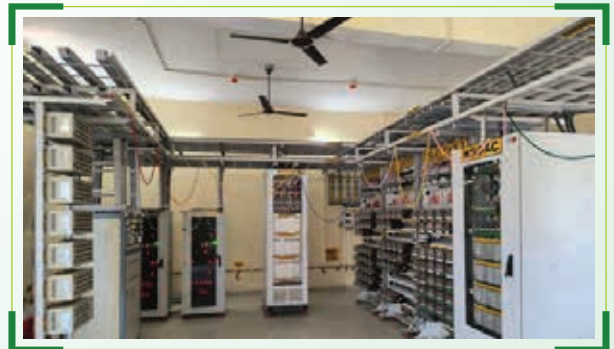
Relay Room, Moradabad S&T Project
