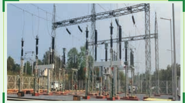
132KV-25KV Badarpur Ghat TSS, RE PKG-2, Lumding Project
