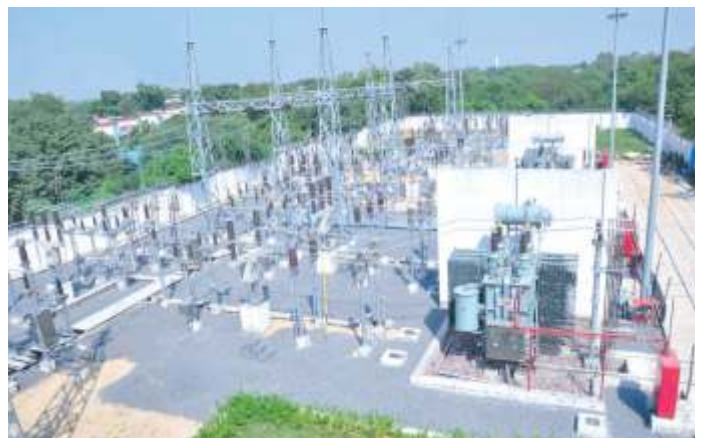
DMRC 66KV Sub Station at INA, Delhi
