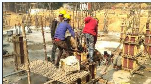
Construction site view of New State-of-Art Building of Department of Science & Technology at Technology Bhawan, New Delhi
