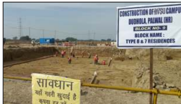
Construction site view of Haryana Vishwakarma Skill University at Dudhola, Palwal, Haryana
