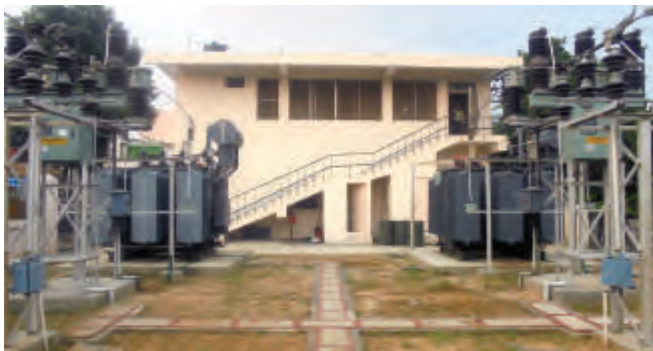
2x5MVA, 33 KV Sub-Station Jagriti Vihar, Meerut
