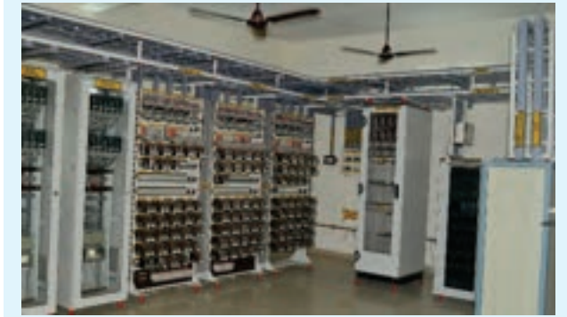
Relay Room Arrangement - Moradabad S&T Project
