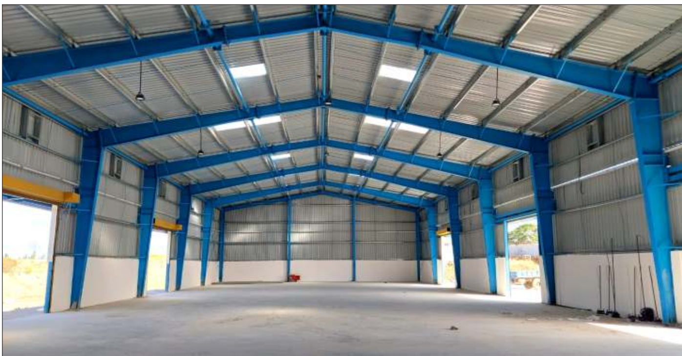
Setting up a Multi Modal Logistic Park (MMLP) at Kadakola Station, Mysuru
