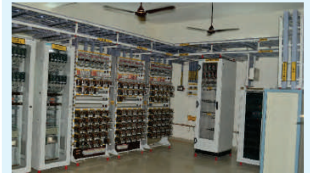
Relay Room Arrangement - Moradabad S&T Project
