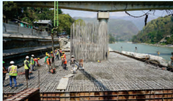
Bridge P P1 Pile Cap Casting in progress-Sivok Rangpo Railway Line Project
