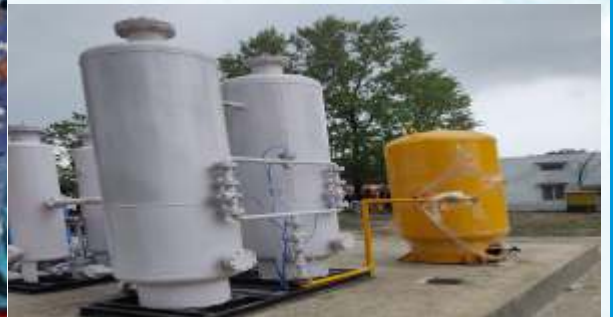
Installation of Oxygen Generating Plant at Divisional Railway Hospital, Samastipur, District of Bihar
